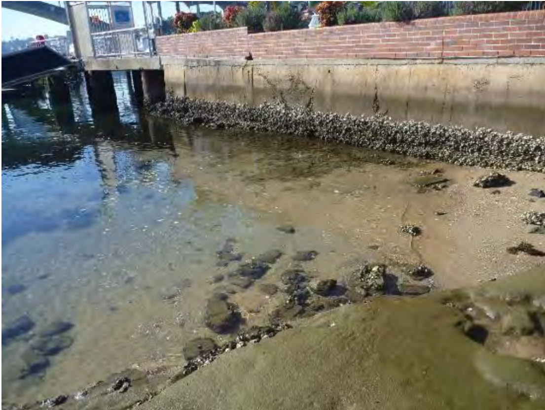
Plate 3: Concrete seawall bounding Gladesville Bridge Marina. Note the dense band of oysters above the waterline.
